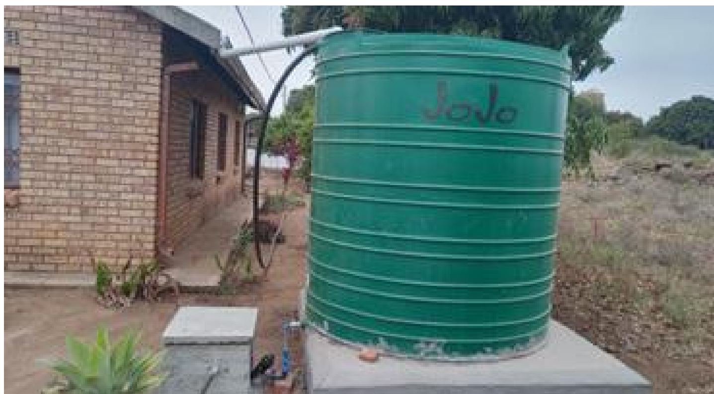
Rainwater harvesting system connected to booster pump
